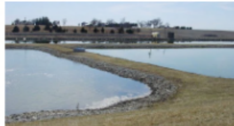
Aerated lagoon system at the wastewater treatment plant in Lenox, Iowa. Read more about this project and more in the Related Technical Experience section.
