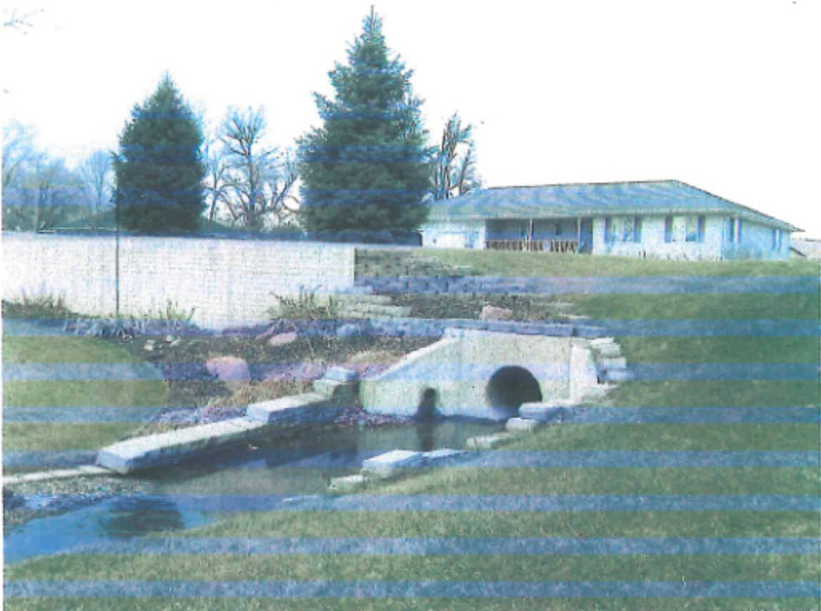
Look north from the utility easement at the outlet from a storm water drainage system that handles the storm water from "E" Street and other streets and properties located in Kozi Addition. Storm sewer outlet is approximately 36" in diameter.
