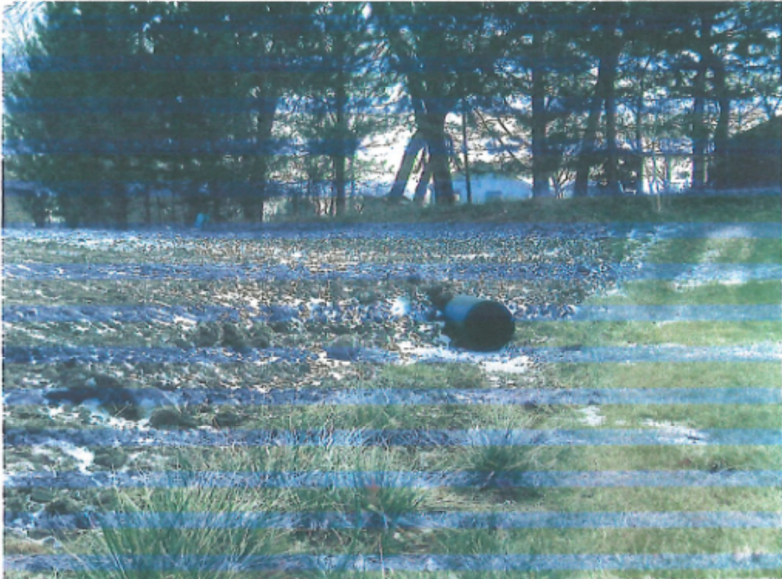
Looking south from the utility easement towards a newly constructed inlet storm water drainage system and dirt fill was installed by or for Patrick and Carol Meysenburg. Inlet is approximately 30" in diameter. Newly constructed inlet storm water drainage system bends or turns to the east to drain into a flowing stream. Before construction, a natural waterway existed in this location.
